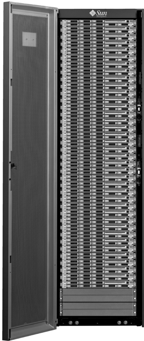
FIGURE 6.15 A standard 19-inch rack populated with 42 1U servers. This rack has 42 1U “pizza box” servers. Source: http://gchelpdesk.ualberta.ca/news/07mar06/cbhd_news_07mar06.php .
